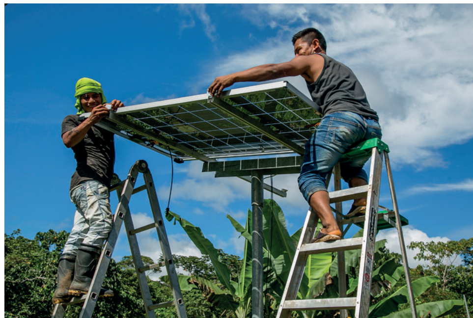
Solar home system installation in the community of Mañoko in the Peruvian Amazon
