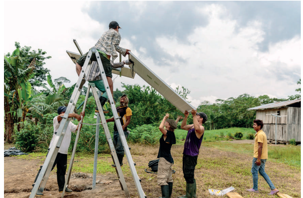
Solar system installation in the Cofán community Bavoroe in 2016.
