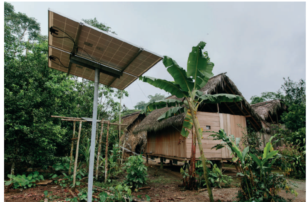
Solar modules on mounting system in the Waorani community Nemonpare.
